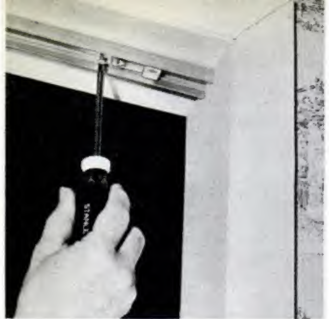
FIRST STEP: Install the overhead track by screwing it to the door-opening header 1 1/2 in. in from edge
